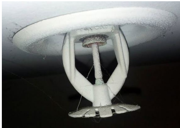
Painted fire sprinkler, by QRFS.com
